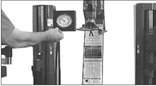
Figure 19 - Location of Manual Release Valve
